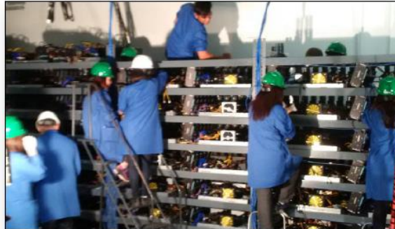
Servers installation phase
