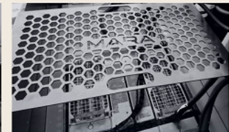
Each tank holds 16 machines
