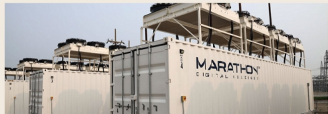
Each custom-built container holds a total of ~128 machines
